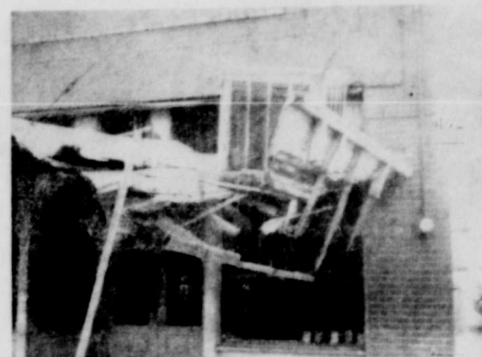
AWNING DAMAGED —The awning attached to the building occupied by Hicks Auto Supply, Ltd., was badly damaged at about 5 a.m. December 20 when a truck crashed into it. An air-conditioning unit resting on the top of the awning was damaged and investigators were of the opinion the entire awning would have to be replaced. No injuries were reported as a result of the accident.
