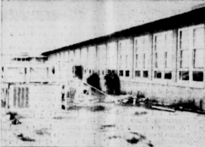
REMODELING THE HIGHSCHOOL. Pictured here is some of the handwork on the Stanton High School during the past months.
