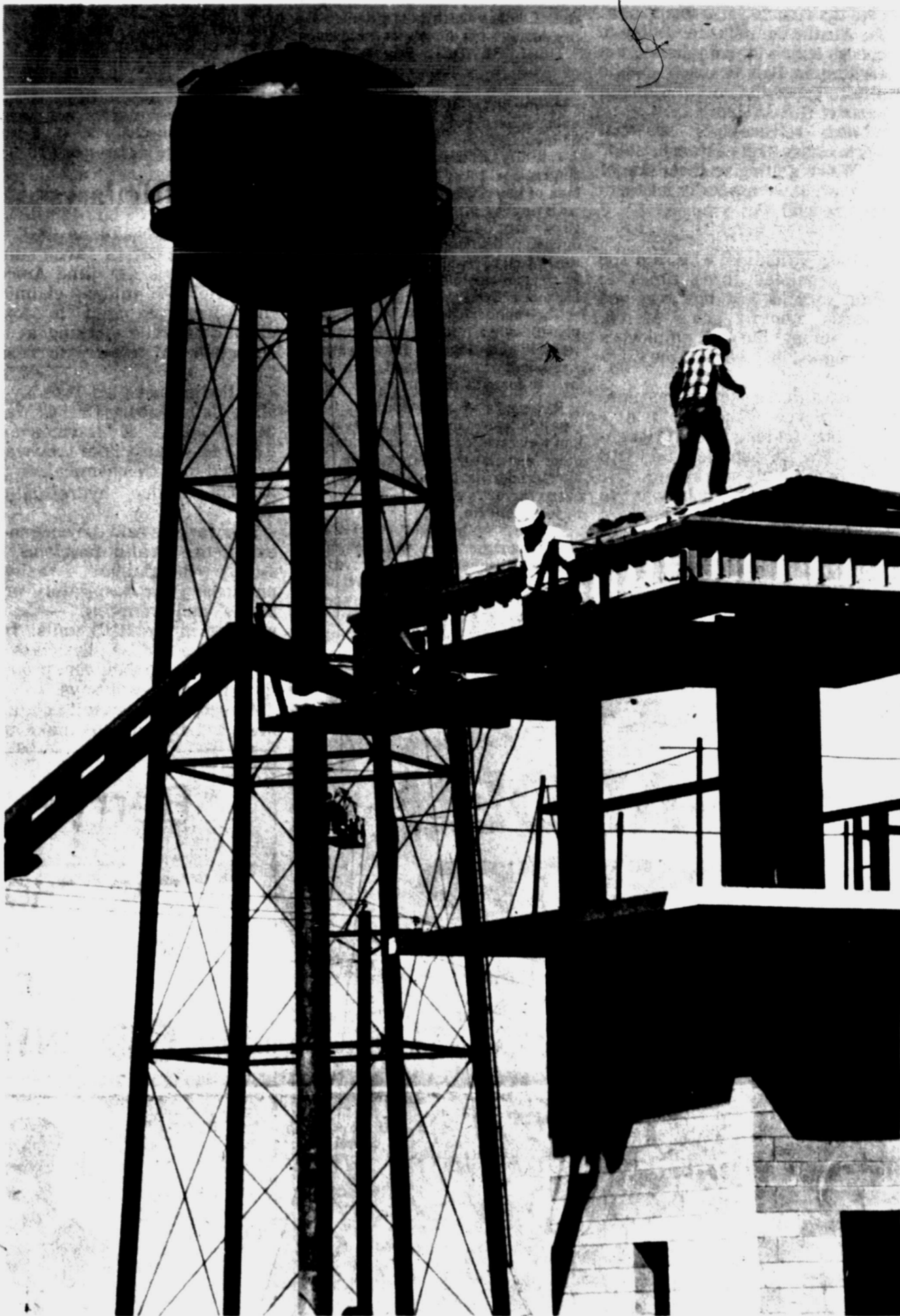
SKY-WALKERS — Workmen at the Price Daniel prison unit are shown finishing a guard tower on the northwest corner of the unit and, in the background, painting the 153 ft. tall water tower, which was erected by Pittsburg Tank & Tower Co. of Pittsburg, Ky. (SDN Staff Photo by Bob Campbell)
