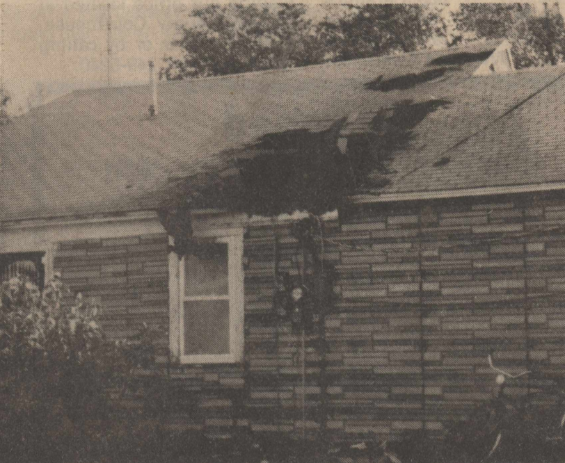
An early morning fire broke out in the attic at 709 N. Poplar, Tues. Sept. 19. No one was home at the time the blaze. It is believed the fire was caused by faulty electrical wiring. Damage was to the roof, attic & two bedrooms of the house.
