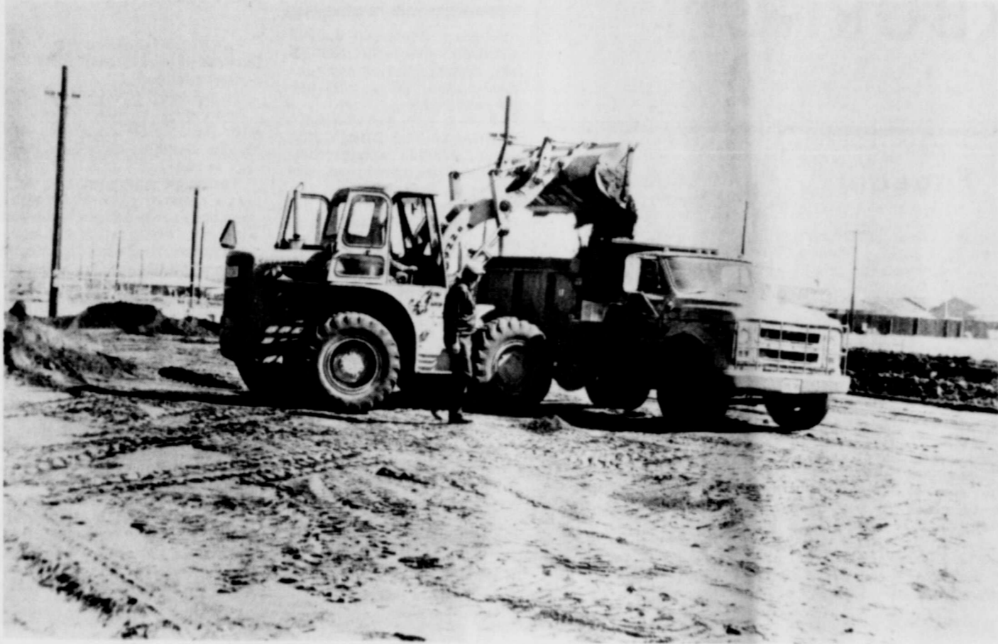
NEW COURTS UNDER CONSTRUCTION---Contractor Joe Ray McCluskey stops workmen for a check on the construction of three new tennis courts at Burk Burnett High School.
