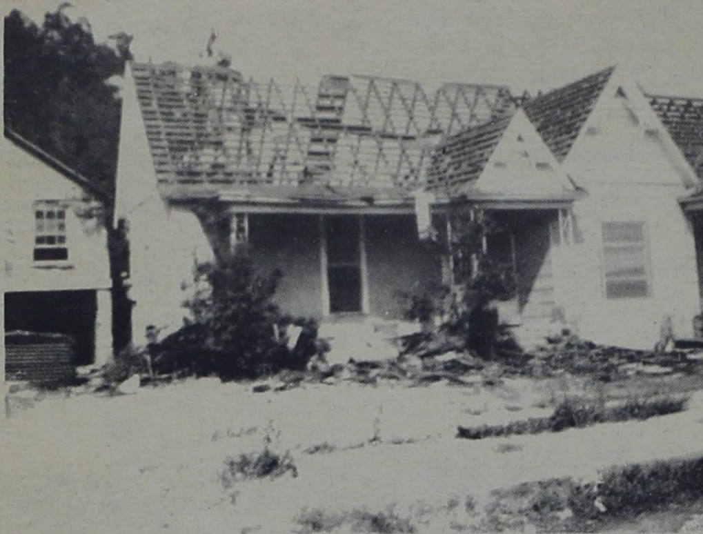
THE OLD GIVES WAY FOR THE NEW— In Sept. 79, Jerry Allen of Baird Electric Inc. starts clearing this lot to make way for a new building, which was Baird Electric Inc.
