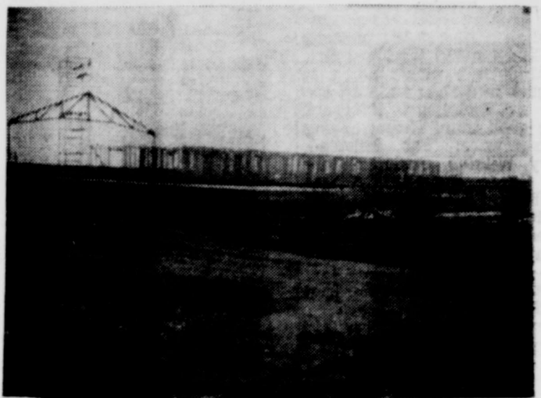
The new First Baptist Church extension, across from the new Junior High School. This building is under construction of Brice Burton Construction Co. Its estimated cost is $100,000.00.
