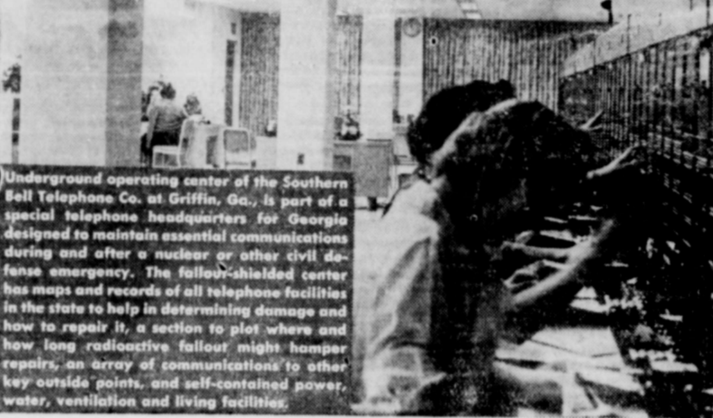
Underground operating center of the Southern Bell Telephone Co. at Griffin, Ga., is part of a special telephone headquarters for Georgia designed to maintain essential communications during and after a nuclear or other civil defense emergency. The fallout-shielded center has maps and records of all telephone facilities in the state to help in determining damage and how to repair it, a section to plot where and how long radioactive fallout might hamper repairs, an array of communications to other key outside points, and self-contained power, water, ventilation and living facilities.
