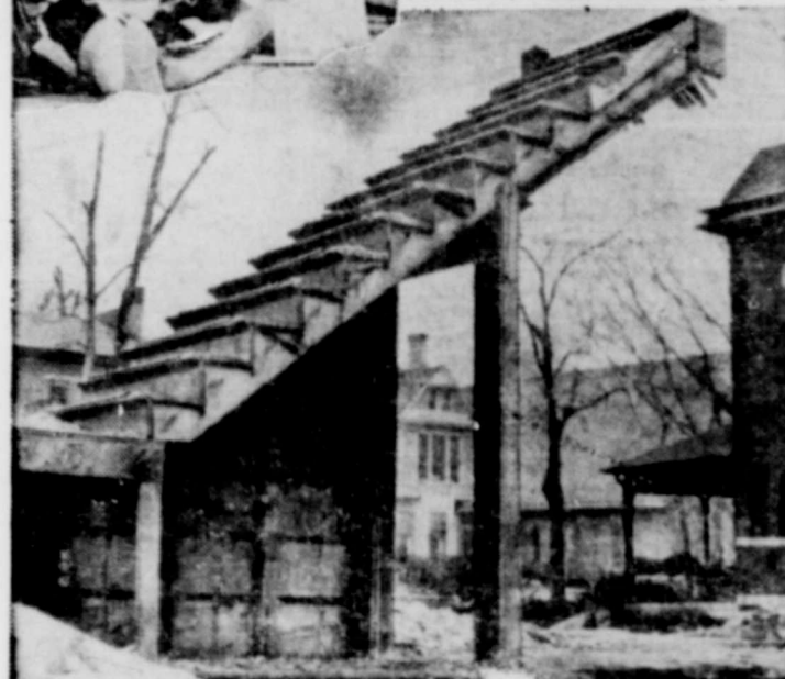
THAT LAST STEP will be a dilly for a jobe using this stairway, all that's left of a house that was torn down in Logansport, Ind.
