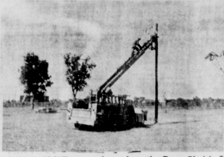
SHOWN ABOVE are workmen from the Texas Electric Co. installing the new lights at the Burk Swim Club Park. The Board of Directors of the Burk Swim Club expressed their appreciation to the City Parks Dept. for their new improvement in the park area. The photo was a courtesy of the Derrick Staff of the Burkburnett High School.
