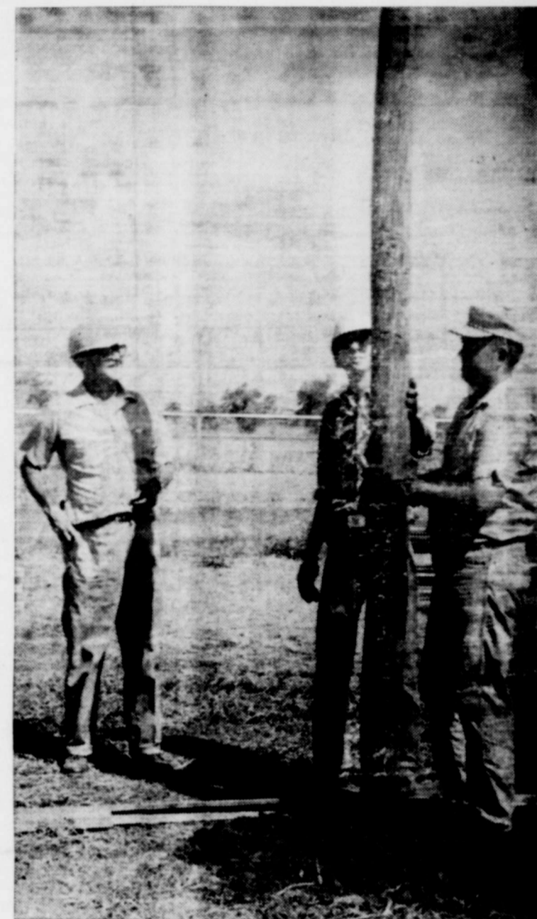
ASSISTANCE in setting up poles at Boomtown, USA Oil Park is provided by James (Sully) Sullivan, Bob Busby and Bill Vincent. The volunteer workers at Thursday's workday made noticeable progress on the park, and enjoyed homemade ice cream as well. Burk Star Photo
