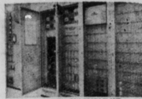
CONTROL ROOM W.T.U. OAK CREEK PLANT
