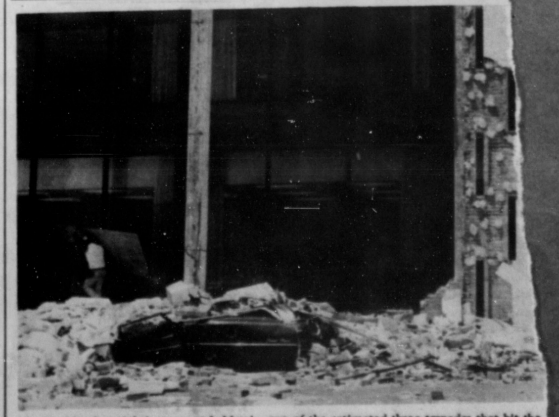
During Monday night's storm at Lubbock, one of the estimated three tornadoes that hit the downtown section pulled huge marble squares from the sides of the First National-Pioneer Building and crushed many cars parked below. The car shown was a new station-wagon but is now about two-feet tall. (Chronicle Photo)
