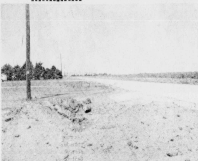
HALE COUNTY Commissioner Henry Rieff reports that repair and topping work has been completed on Abernathy's Cemetery Road. The county saved a considerable amount of money by having county employees fill the pot holes and other damaged spots before having a contractor put on the new topping.
