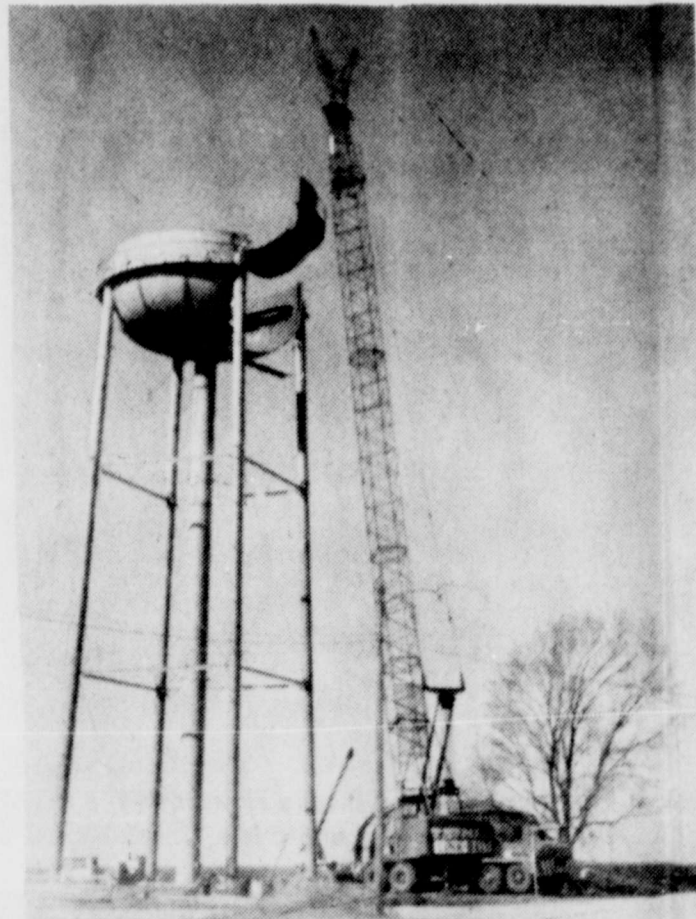
HUMPTY DUMPTY—Universal Tank and Ironwork daring crew succeeds where "All the King's horses and all the King's men" failed—putting our giant new water tower together—just like Humpty Dumpty, only better.
