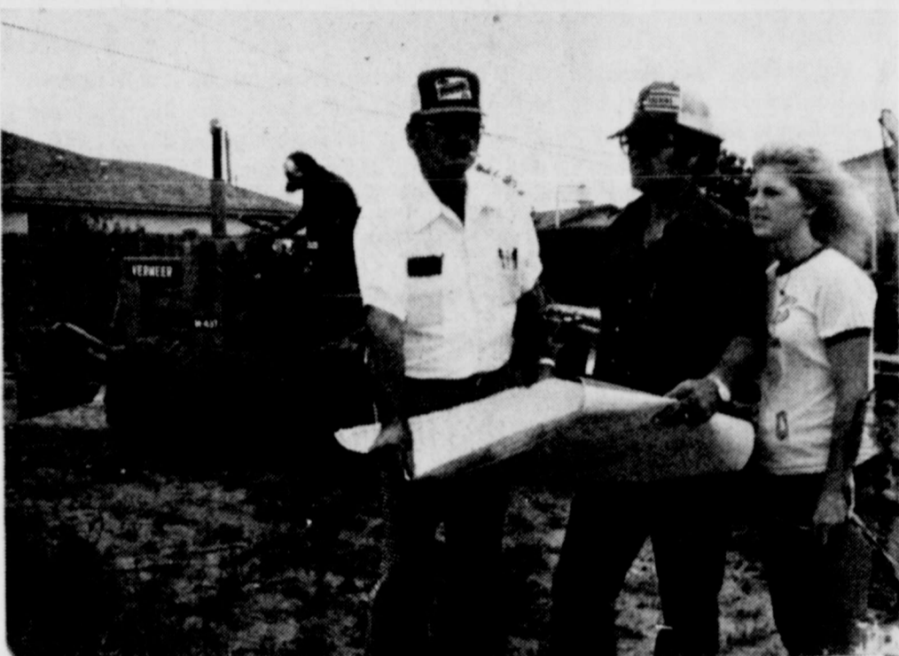
CABLE GOING IN - Billy Gist and daughter Cherise (center and at left) check cable TV installation plans with Jesse Morrison of Panhandle Cable TV. H.L. Robertson operates the trench digger behind them.
