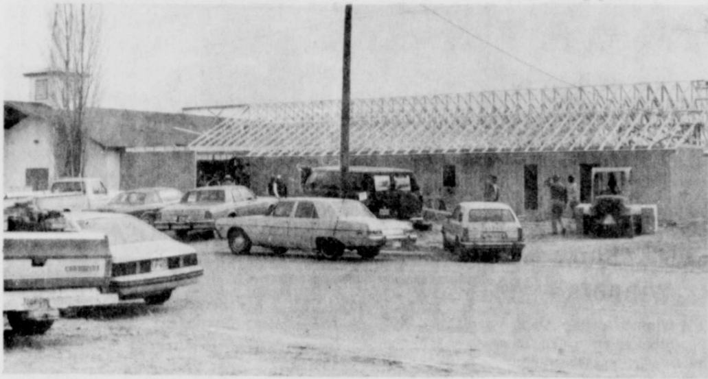
PRIMEIRA MISSION BAUTISTA being added onto this past week by volunteers from everywhere. (Review Photo)
