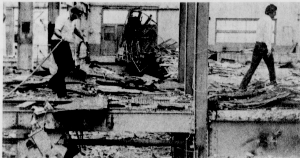
A FIRE STARTED at the old Tuco Plant when some piping ignited while welders were at work. Pictured are firemen Tom Conway and Ken Hendrix.
