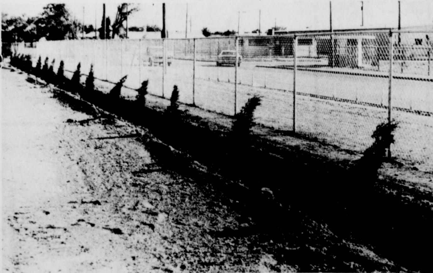
JUNIPERS AND FENCES were installed recently around the two lots located just west of the elementary building. A gate has been left open for children to use the playground equipment. (Review Photo)
