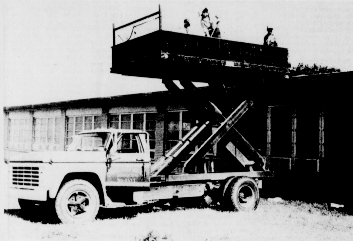
A GRAVEL AND TAR coating was put on the roof of High School Friday. Pictured are employees of Lydic Roofing Company shoveling gravel from the bed of this lift truck onto the roof. (Review Photo)
