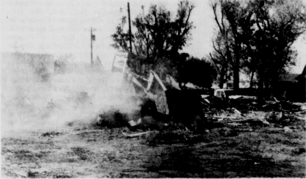
BUILDING REMOVED that stood on the 1000 block of Ave. D. It was a substandard building and was condemned by the City. A building was also removed from the Methodist Church lot last week. (Review Photo)
