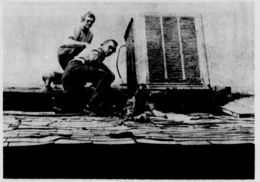
ABERNATHY FIREMEN investigate a small fire in the attic of Abernathy Meat Products, located on the northeast side of town. The fire was thought to have been caused by a short in the wiring. (Review Photo)
