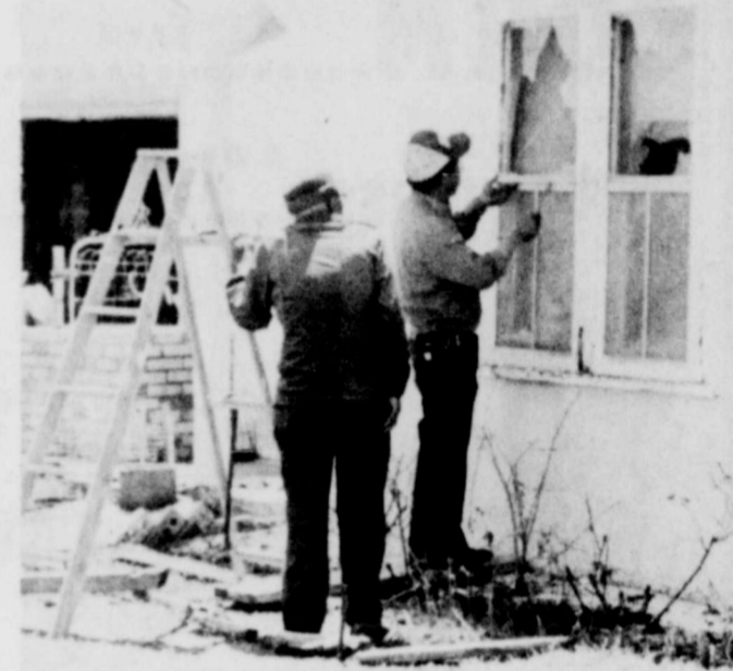
BROKEN WINDOWS all over town following the storm last Tuesday night. In the top photo, a boy observes broken windows in his house. In the bottom photo, two men repair a set of windows. (Review Photo)
