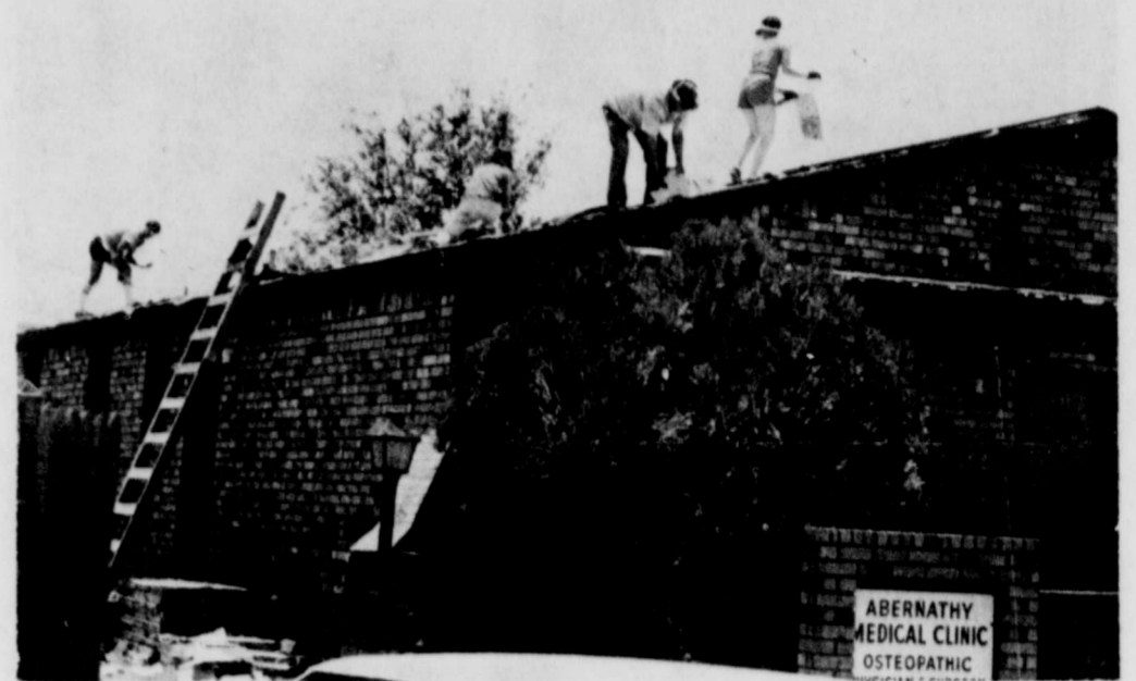
ROOFING TAKING PLACE at a rapid pace in Abernathy following a storm which destroyed roofs in Abernathy a month ago. Pictured are roofers working on the Abernathy Medical Clinic roof. (REVIEW PHOTO)
