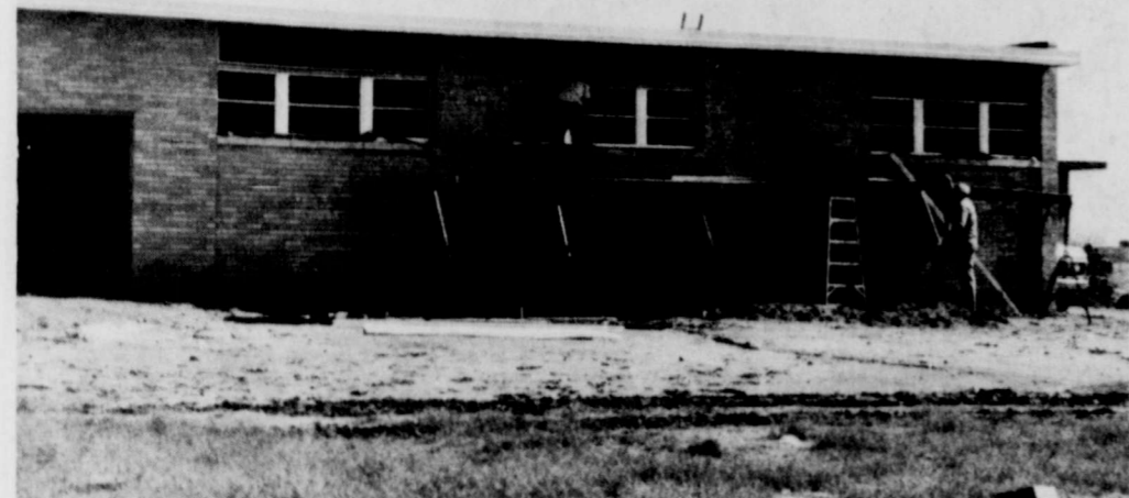
SHALLOWATER SCHOOLS continue to grow. New athletic dressing room facilities became necessary when the number of students participating in athletics outgrew the present facilities. The structure will be completed by the opening of school, if the weather will cooperate. (Review Photo)
