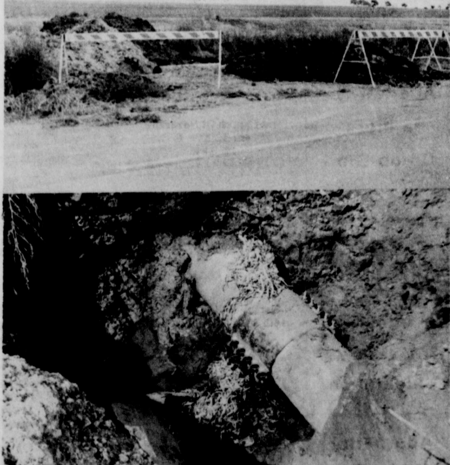
BREAK IN WATER LINE which supplies water to Abernathy residents occurred last week. It took a crew half a day to dig it up and seal it. In the top photo is where the leak occurred, approximately five miles east of town on highway 597. In the bottom photo, is a large clamp placed around the pipe to keep it from leaking. The line was fixed before city residents ran out of water. (Review Photo)
