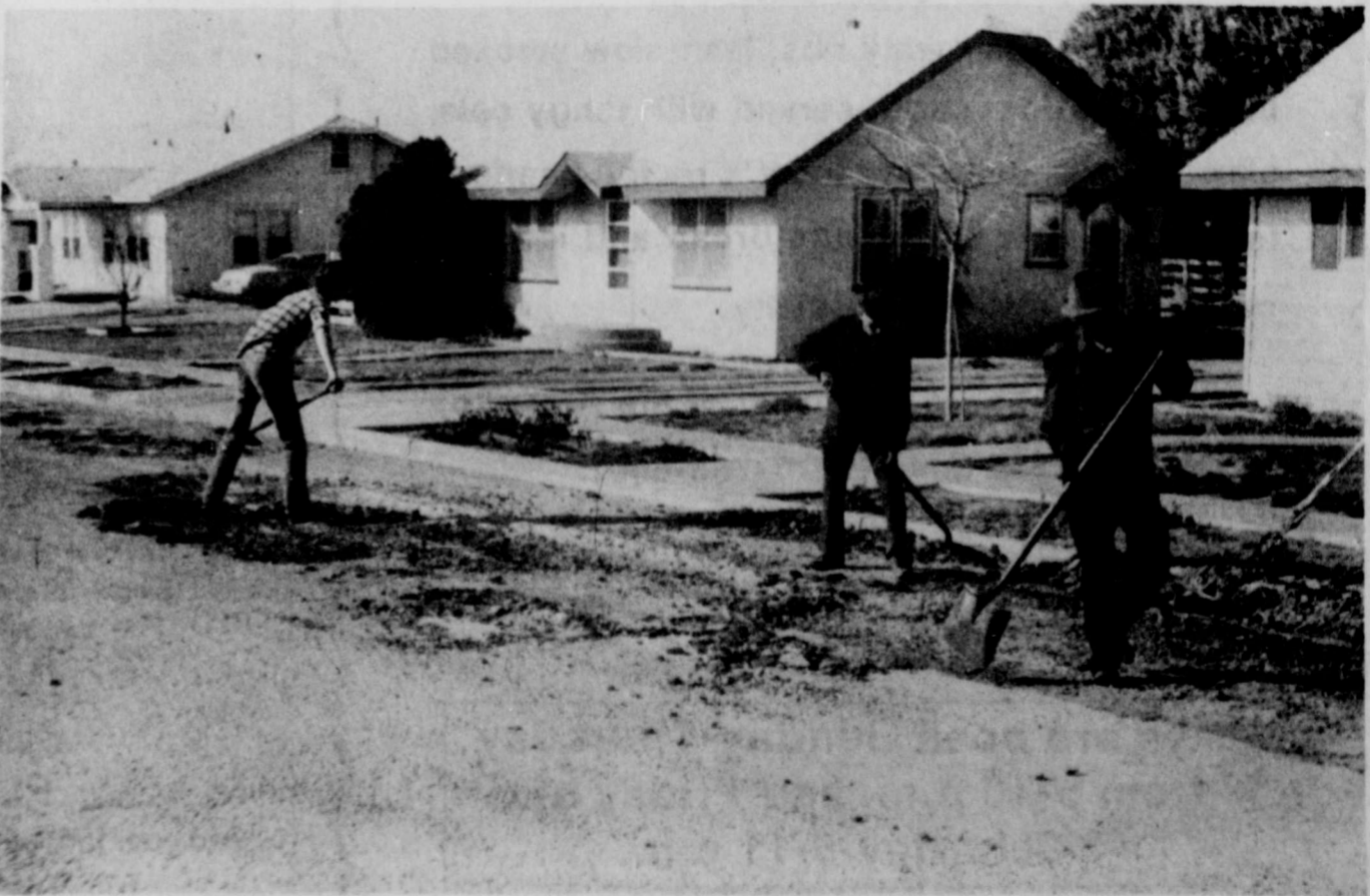
CITY STREETS BEING REPAIRED all over town after the two weeks of cold weather and snow on the ground. The freezing slush damaged many city streets with chug holes. (Review Photo)
