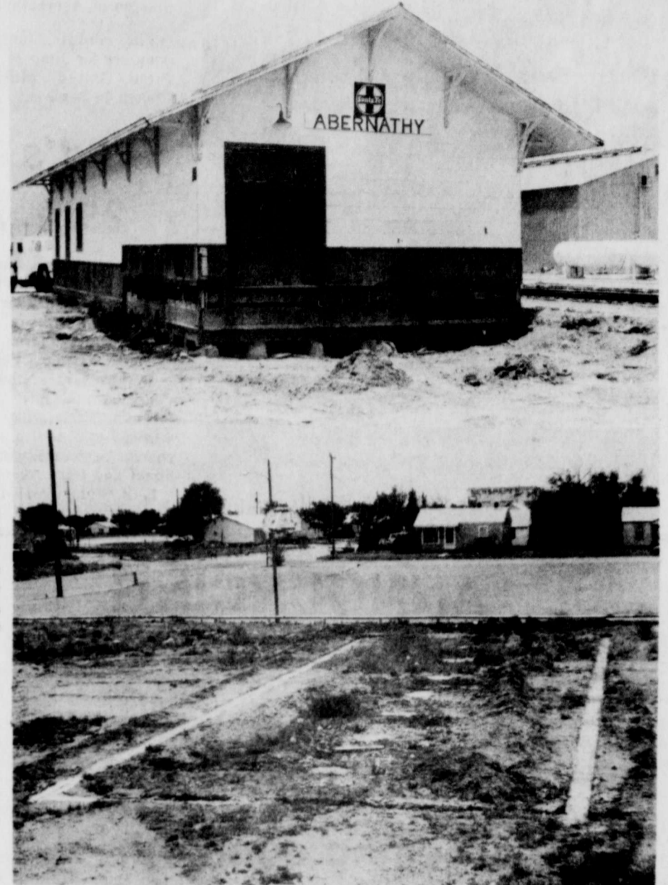
OLD AND NEW LOCATIONS for the Santa Fe Depot (future Senior Citizens Center). In the top photo is the depot after a crew removed the loading platform from around it this past weekend, so it can be moved. In the bottom photo is the new location, just north of the Methodist Church parking lot. Pictured is the cement footing. (Review Photos)
