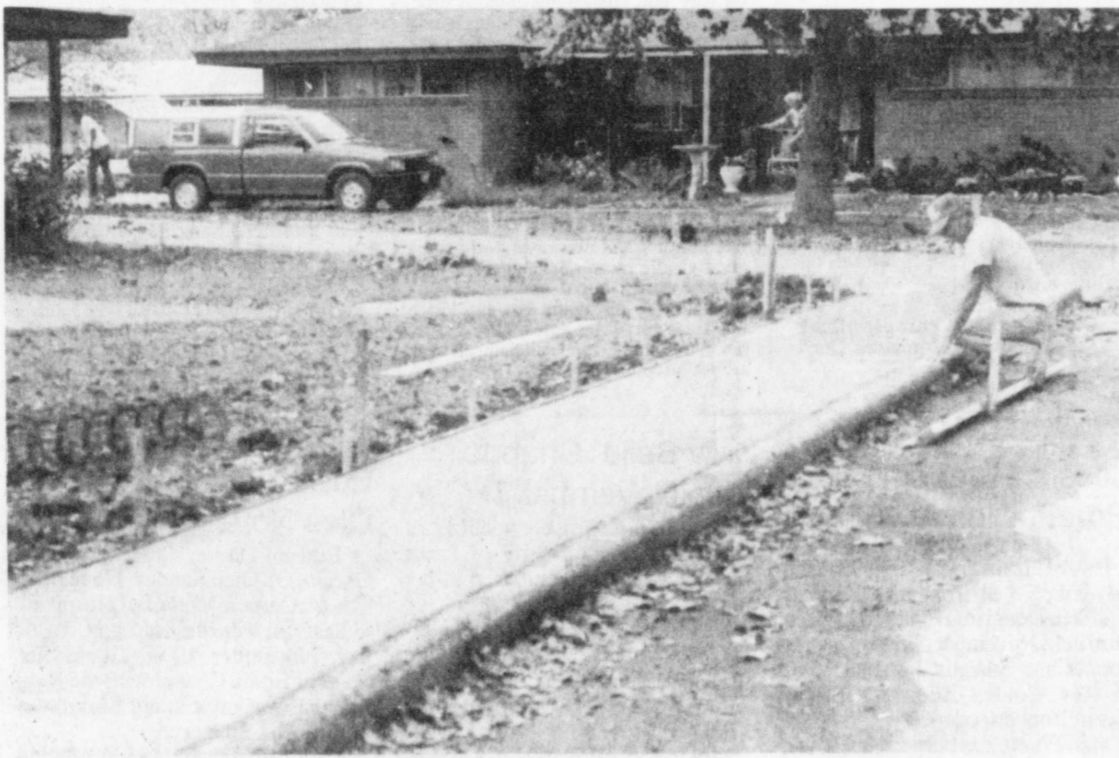
NEW SIDEWALKS -new concrete was poured last week at the Deport Housing Authority
