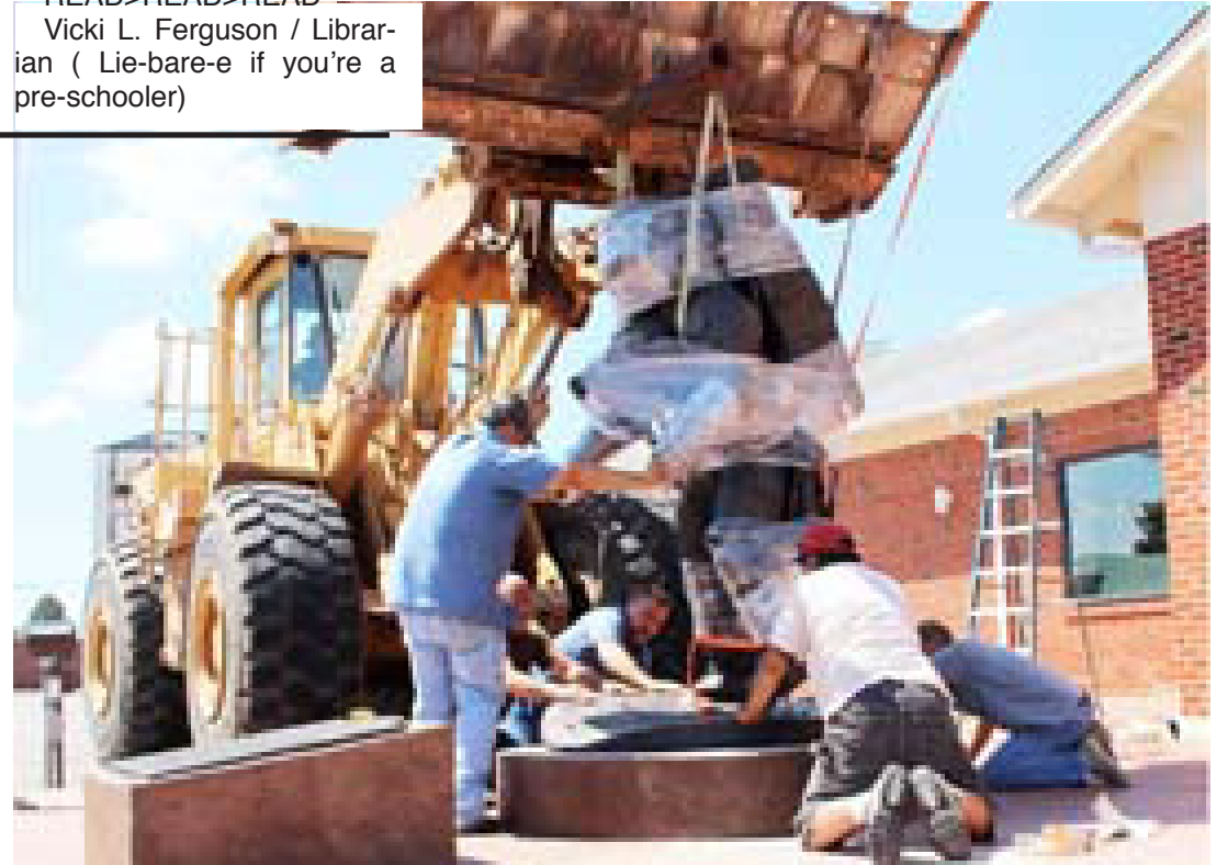
STATUE: The Alan L. Bean statue was delivered Monday morning. The county and city employees were called in to help. Shown here are Jimmy Don Brown (driver), Paul Arganbright, Bobby Jones (Bobby Jones Welding), Chip Hill (RiverCrest Concrete), Josh Couch and Victor Loera.
