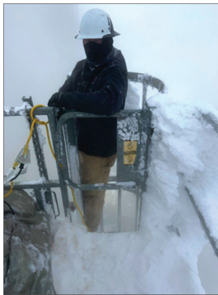
SEVERE WORKING CONDITIONS: This is a photo taken last month of Mike Harz, instrument working foreman at Xcel Energy's Harrington Generating Station northeast of Amarillo, removing ice and snow from an ash silo at the Harrington plant during Winter Storm Uri.
