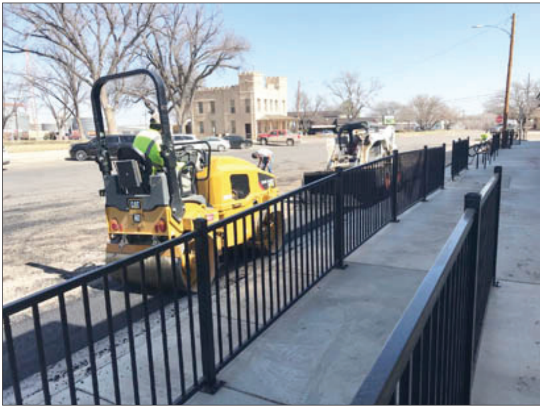
FINISHING TOUCHES: The asphalt was pressed into place last Thursday, as the finishing touches are added to the Texas Street Sidewalk Project.
