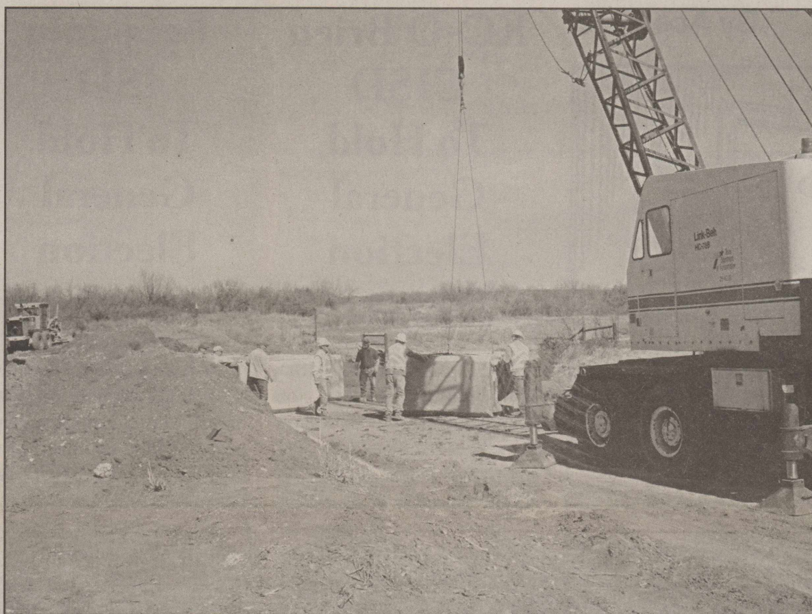
Texas Department of Transportation (TxDOT) crews put in a crossing made of concrete culverts, fill dirt and milled highway at the Croton Creek crossing.
