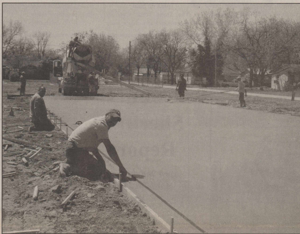
Gabriel Cordova of Tomas Concrete Construction works on the concrete slab of Baize Self-Storage
