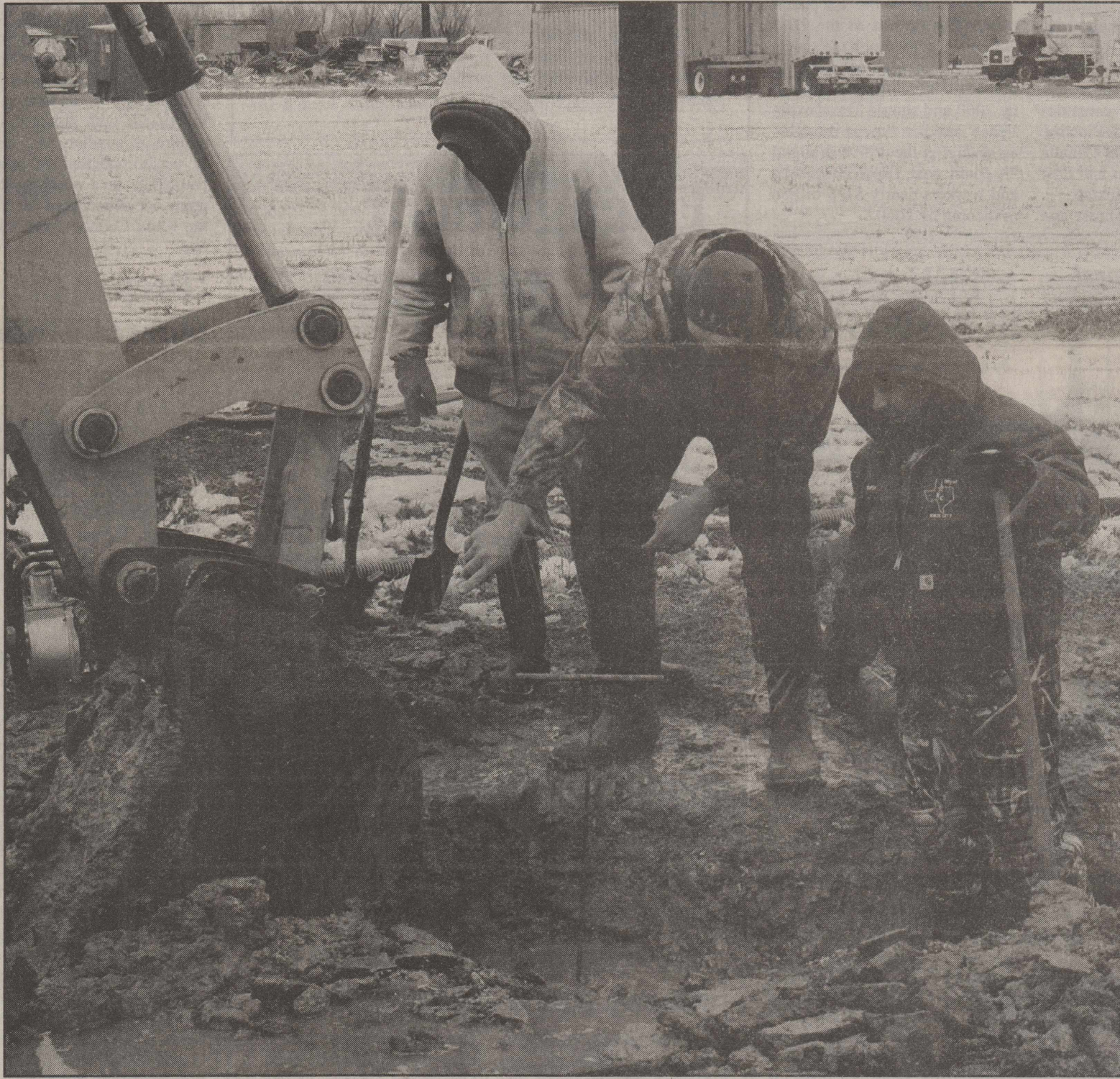
Knox City administrator Chad Roberts (center) points to a place where a problem with one of the city's water lines occurred on Monday. City employees, battling cool temperatures, snow and lots of water, used a backhoe to excavate the ground around the break.
