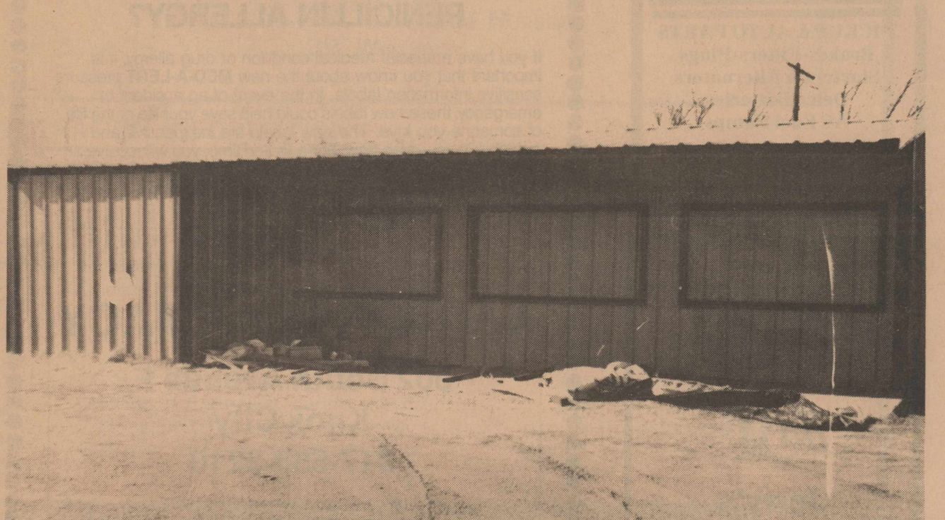
A NEW CONCESSION STAND and new restrooms are a part of the construction taking place at Greyhound Stadium that also includes a modern, up to date track facility. The new work will give Knox City sports fans the convenience of a concession stand and rest rooms located just north of the field house. (News Photos)
