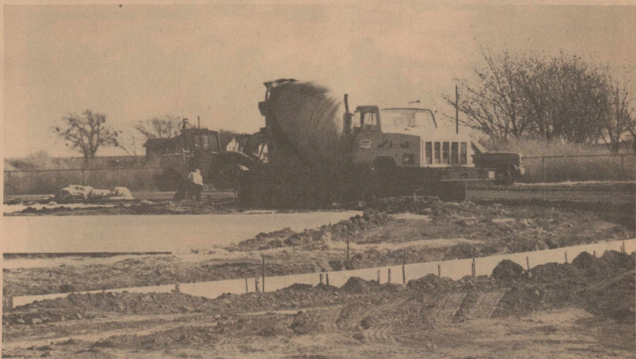
CONSTRUCTION CONTINUES on the new track facility being erected at the Knox City High School Football Field. The new work at Greyhound Stadium will allow Knox City to host District Track Meets and is being constructed with no tax increases to local taxpayers. (News Photo)
