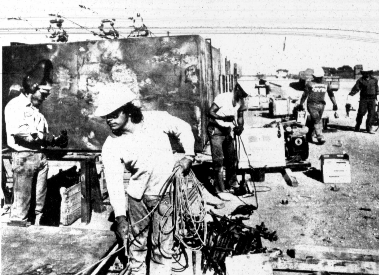
WELDING — Welder Tony Bartlett, left, and Raymond Aguilar, foreground, both of San Marcos, last week were working on the cell forms that will be used at the Texas Department of Corrections' new unit east of Snyder. (SDN Staff Photo)
