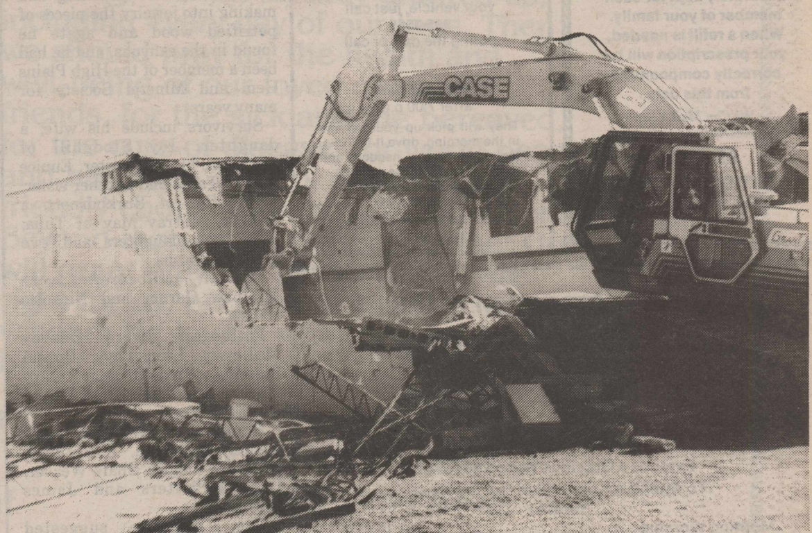
Grant Construction Company ripped through the first section of the old field house last Thursday, and has been in the process of removing rubble from the site before the next demolition takes place. Dirt from the digging of the basement eventually will be used to level the site before new construction begins. School administrators are hoping for completion of the new field house about August 1.
