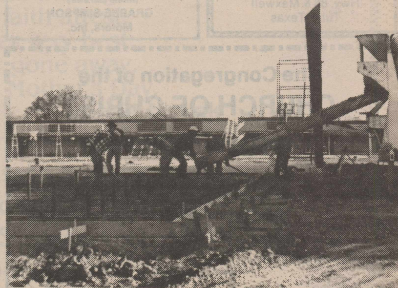
The steel framework for the walls of the new PE Gym is going up on the schoolgrounds this week.
