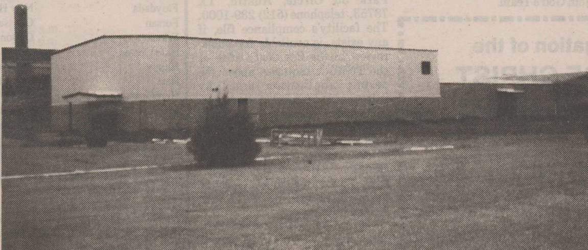
The new PE gym and fieldhouse have taken form quickly and are moving on toward completion. Work has been continuing inside and the area outside is being cleared and leveled so the parking area can be prepared for use by football fans during the upcoming season. Briscoe County News Photo
