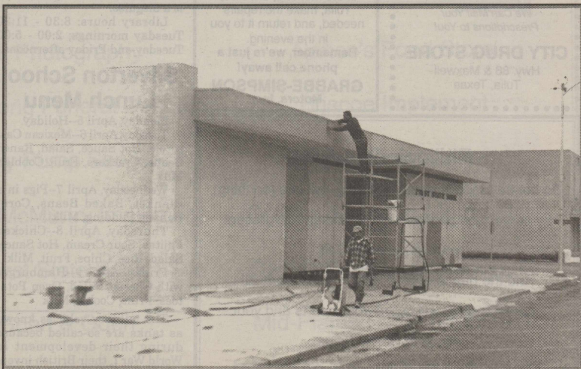
Work is continuing on the facade of First State Bank. The remodeling that is underway will probably continue for several more days, and at some time may require that customers enter the bank through the Pioneer Room.
