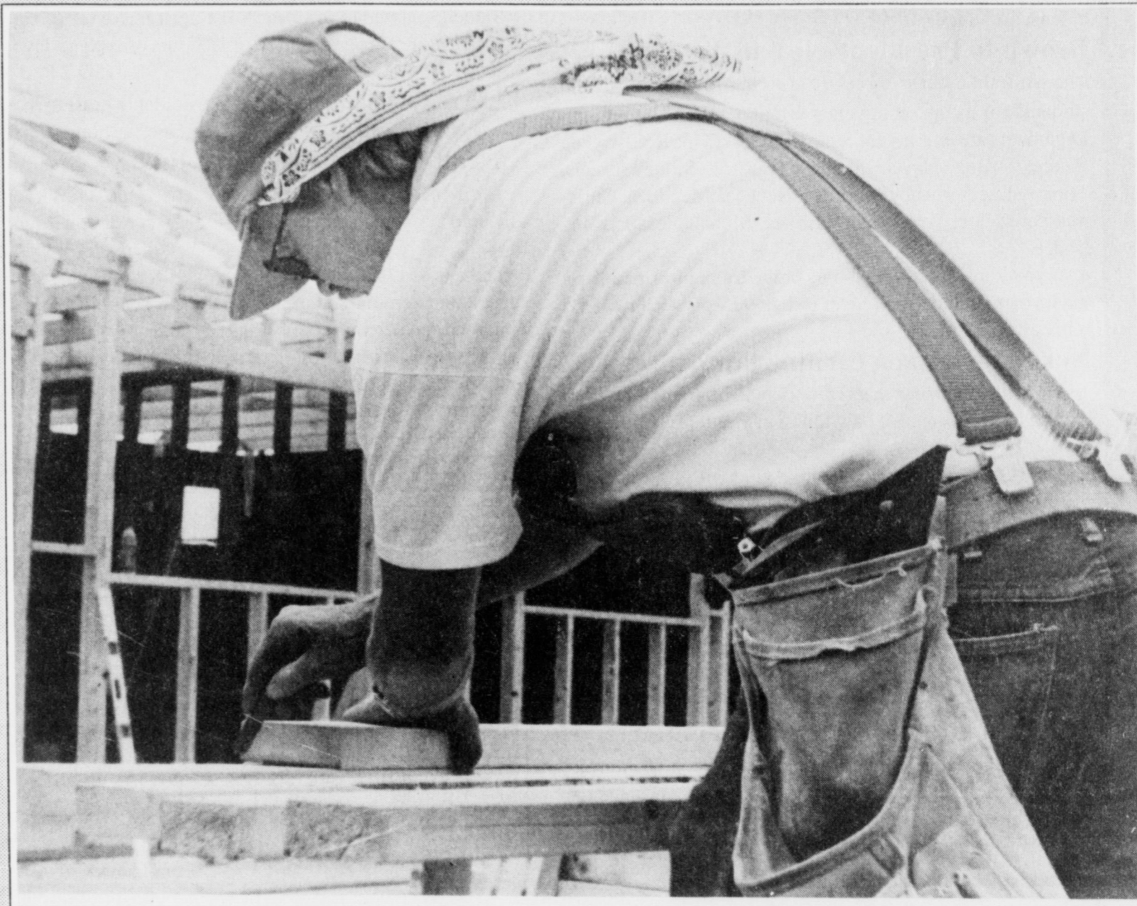
Richard Doran of Preferred Painters of the Southwest, Inc. of Clovis cuts 2x4s Thursday while working to rebuild the Valley Motel. The motel was partially destroyed during a May fire.
