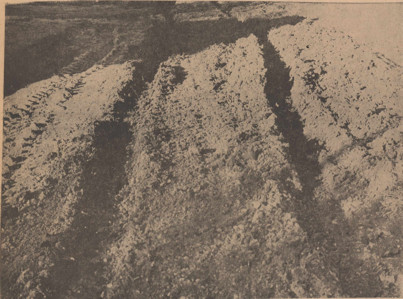
This picture was taken Tuesday and shows the block of Second Street between Main and Avenue E. After a light shower this street is almost impassable. Olton's need for paving and repair of existing paving is acute at the present
