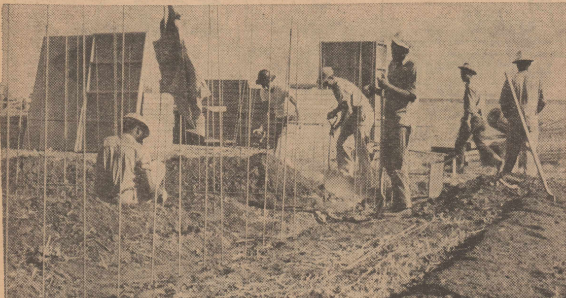
Workmen are shown here beginning construction on the new $25,000 Olton Farm Supply building. It is to be erected on Highway 70 in west Olton. It will parallel the highway with a frontage of 121 feet. (PERSONAL PHOTO)
