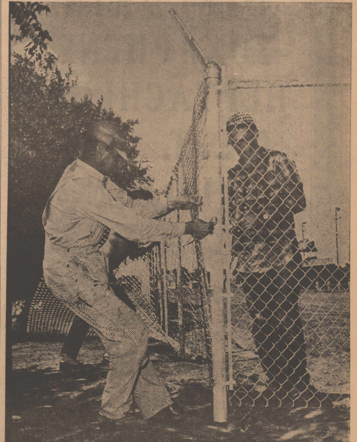
A new cyclone fence is being erected around the football field and athletic area. Workers are shown here putting the finishing touches on the southwest corner of the fence. The improvement also includes a ticket house.
