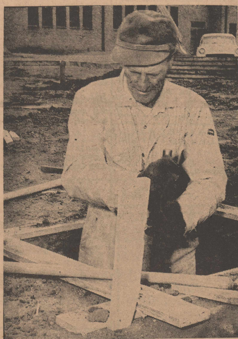
E. H. Teal is shown here working on the foundation of Olton High School's new $200,000 gymnasium. Brick work has started on the elementary building.
