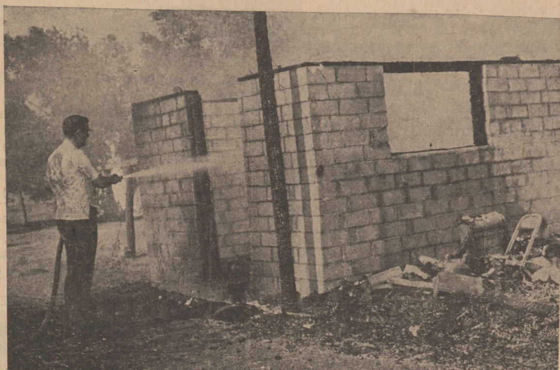
Lynn Fite is shown here spraying a fire which damaged a garage at the Roy Thurman place, 5 miles south of town. The fire is believed to have been started by sparks from a cutting torch.
