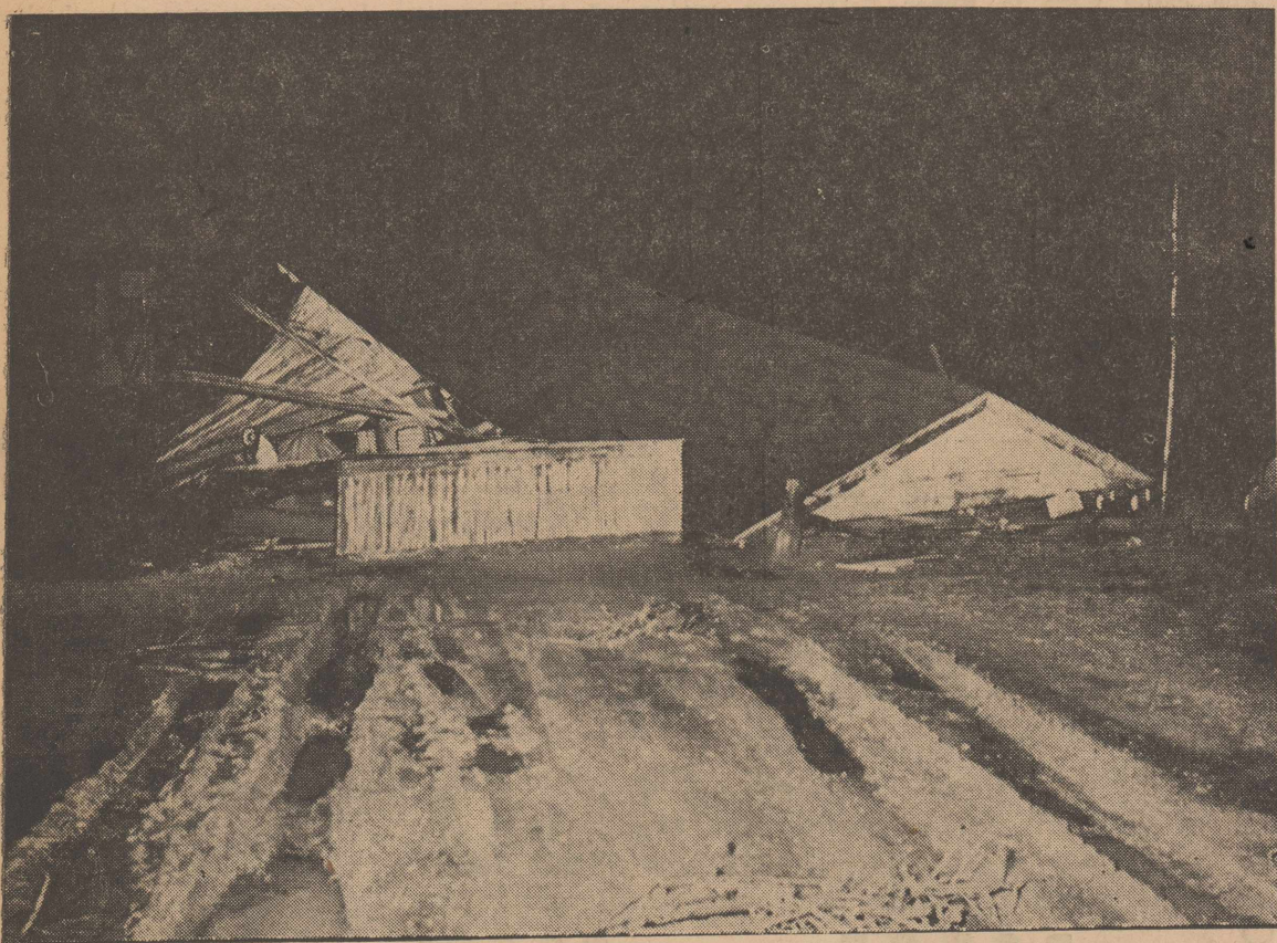
This shambles is what was left of the garage at the Eddie Moore home after it was struck by high wind Wednesday night. Night Officer David Maxey believes east Olton was hit by a tornado. (STAFF PHOTO)
