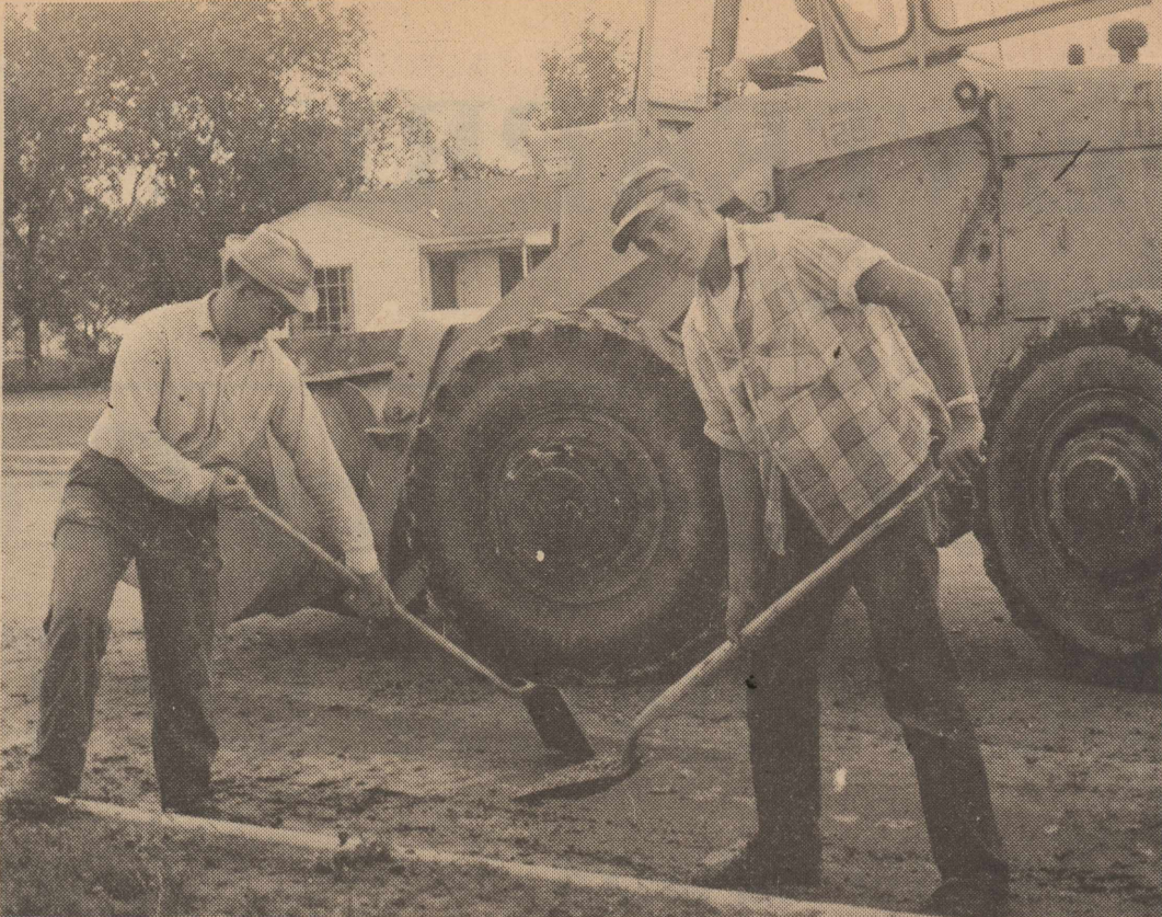
PAVING PROGRESSES--These two workers battled mud last weekend so paving contractors could prime coat roads. After rain continued, paving work was stopped Monday but resumed Wednesday. The paving project is expected to be completed in about three weeks.
