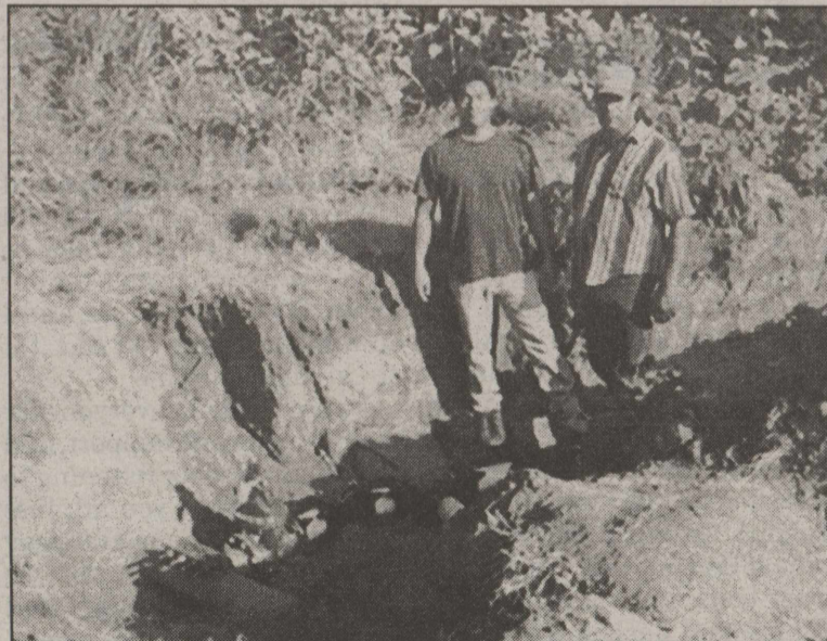
Norberto's Backhoe & Irrigation has been laying a waterline from the City of Quitaque to Caprock Canyons State Park. The water meter has been installed and was inspected Wednesday of last week. Norby and Norberto Garcia were pictured at work.
