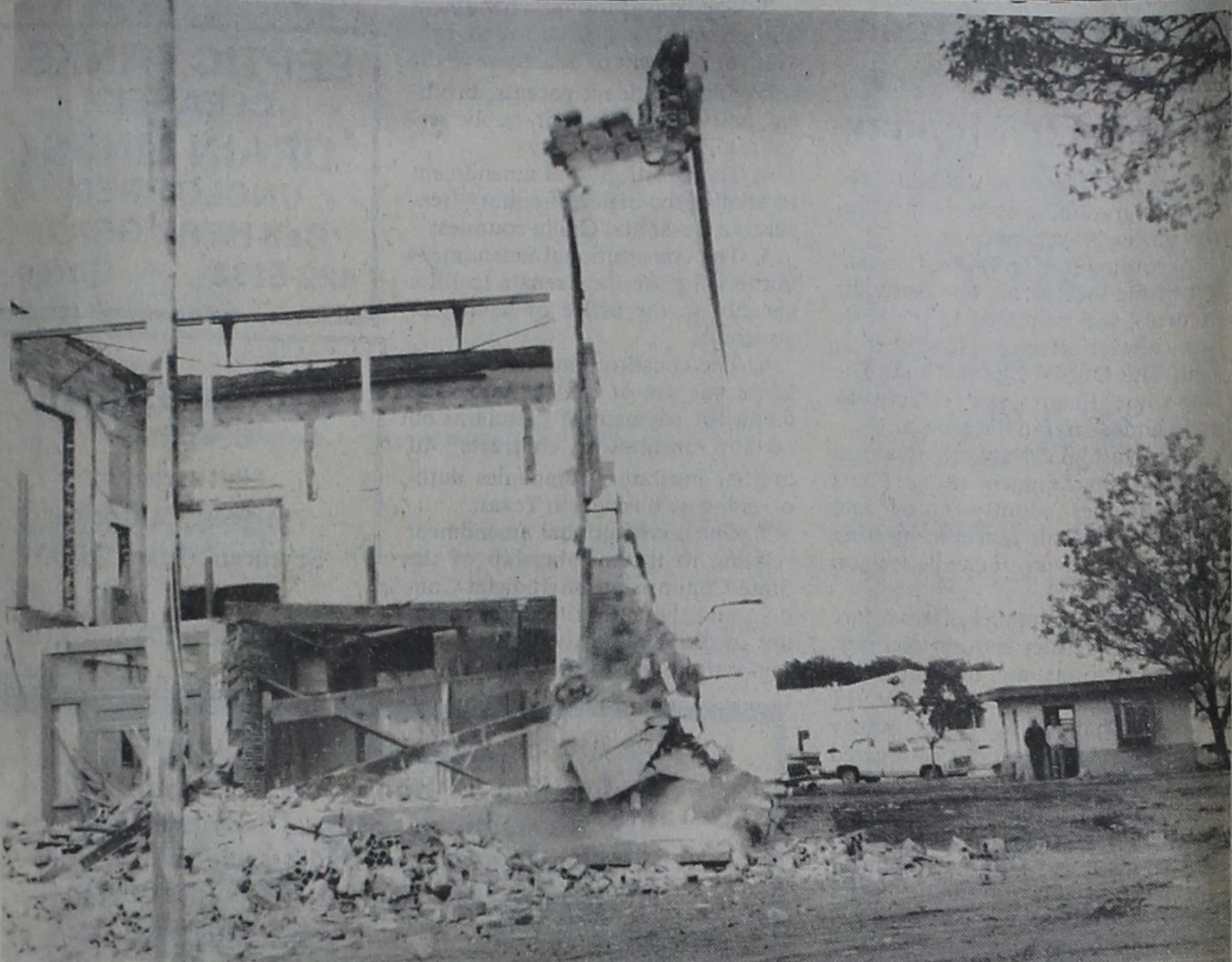
A DESOLATE SIGHT INDEED is this remaining portion of the old Munday City Hall. Interior stripping had been completed with only the shell left when workmen
